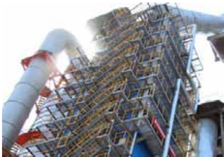
Exhaust heat power facilities (Yantai)
